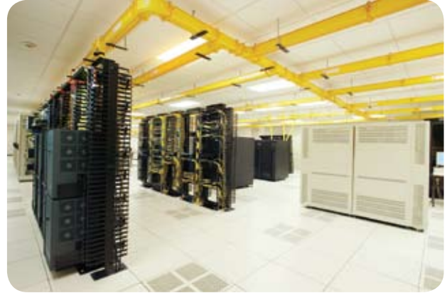
Figure 1. Data Center with Flexible White Space
